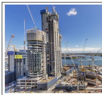
The International Towers Sydney office buildings under construction. (Image courtesy of BDA)
