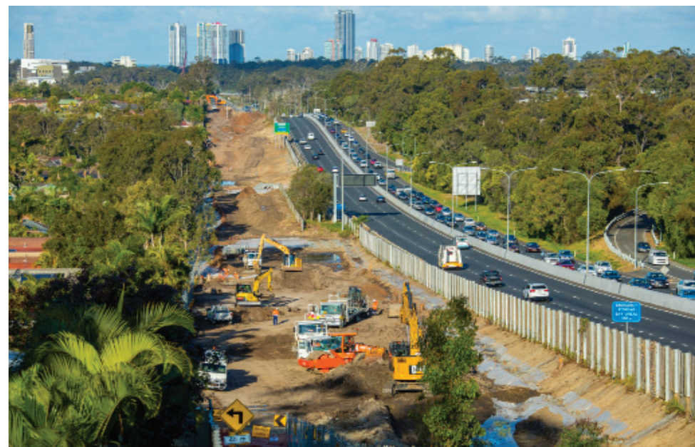
The Gold Coast Light Rail Stage Two under construction – Smith Street looking east.
